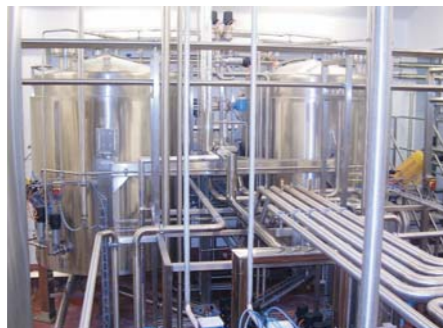
Powder Addition System
