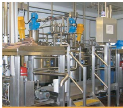
Preparation Mix Plant
